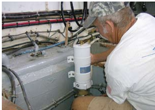
SUPPLY SIDE. New fuel filters and supply lines go in before the new engines.
